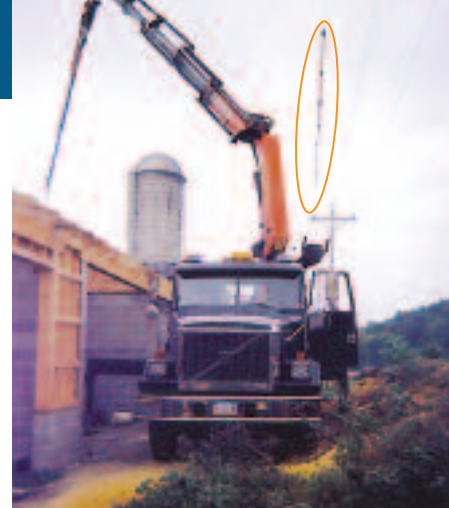
SAFETY FIRST: Special cover-up material is used to cover energized lines to prevent an accident. This cover-up was placed on the wires once the cooperative was contacted.
